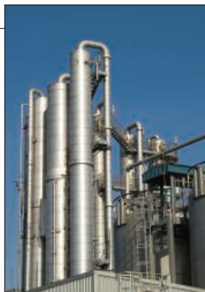
FIGURE 1. This photo shows the EOEG plant at Reliance, Dahej Manufacturing Division
